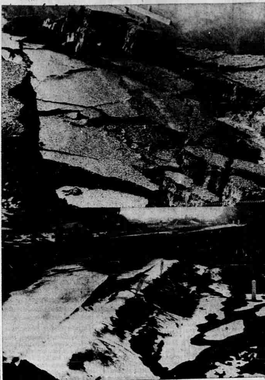
Top view shows six foot settlement in Northwest Coast street, Newport, immediately north of Nye beach. Settlement here may be attributed to erosion of a soft sand base over which the road was built. Lower: Settlement of the highway near Buell on Wallace bridge cutoff is due, say state highway engineers, to a slip plane formation well lubricated by long winter rains. A new, realigned section of highway will be constructed to the northward to bypass this slip plane formation.
