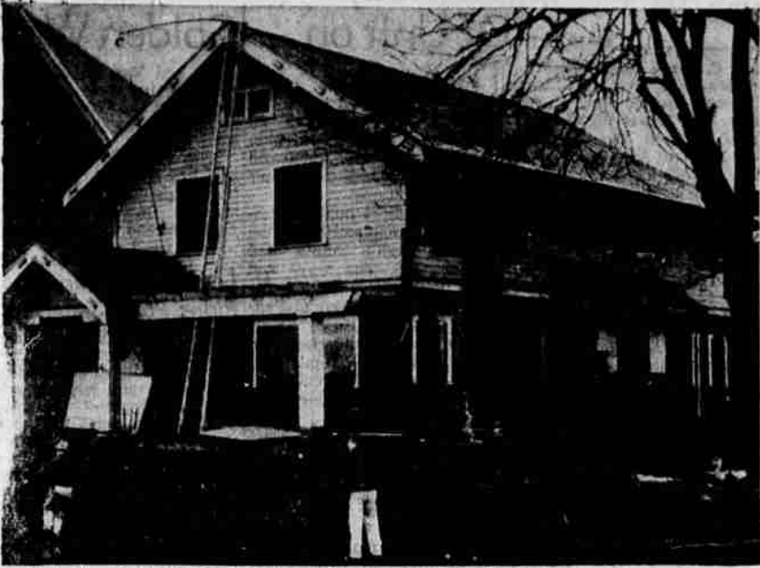
Shown is the former Episcopal rectory as it reached Chermeketa street Friday morning enroute to its new location at Davidson and Lefelle Streets. Allstate Construction company, Portland movers, supported the bulky structure upon 24 wheels on its journey a mile southward to its new location.
