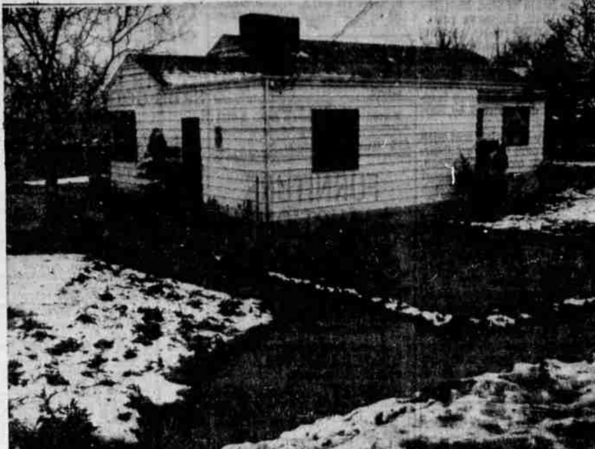
Shown is the home of Don Dill, 975 Morningside, as it appeared Wednesday morning as improperly drained water approached the floor level. Dill believes a drainage line, clogged or fractured by last summer's street improvements made under county supervision, may be responsible for the small geyser spouting from a catch basin at his curb.
