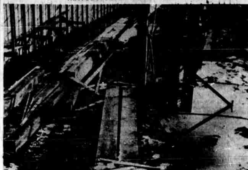
Melting snow in the excavation of Lipman's store basement created this aspect Monday morning when construction workers arrived to pump out water and went slogging through the mud preparatory to placing heavy timbers.
