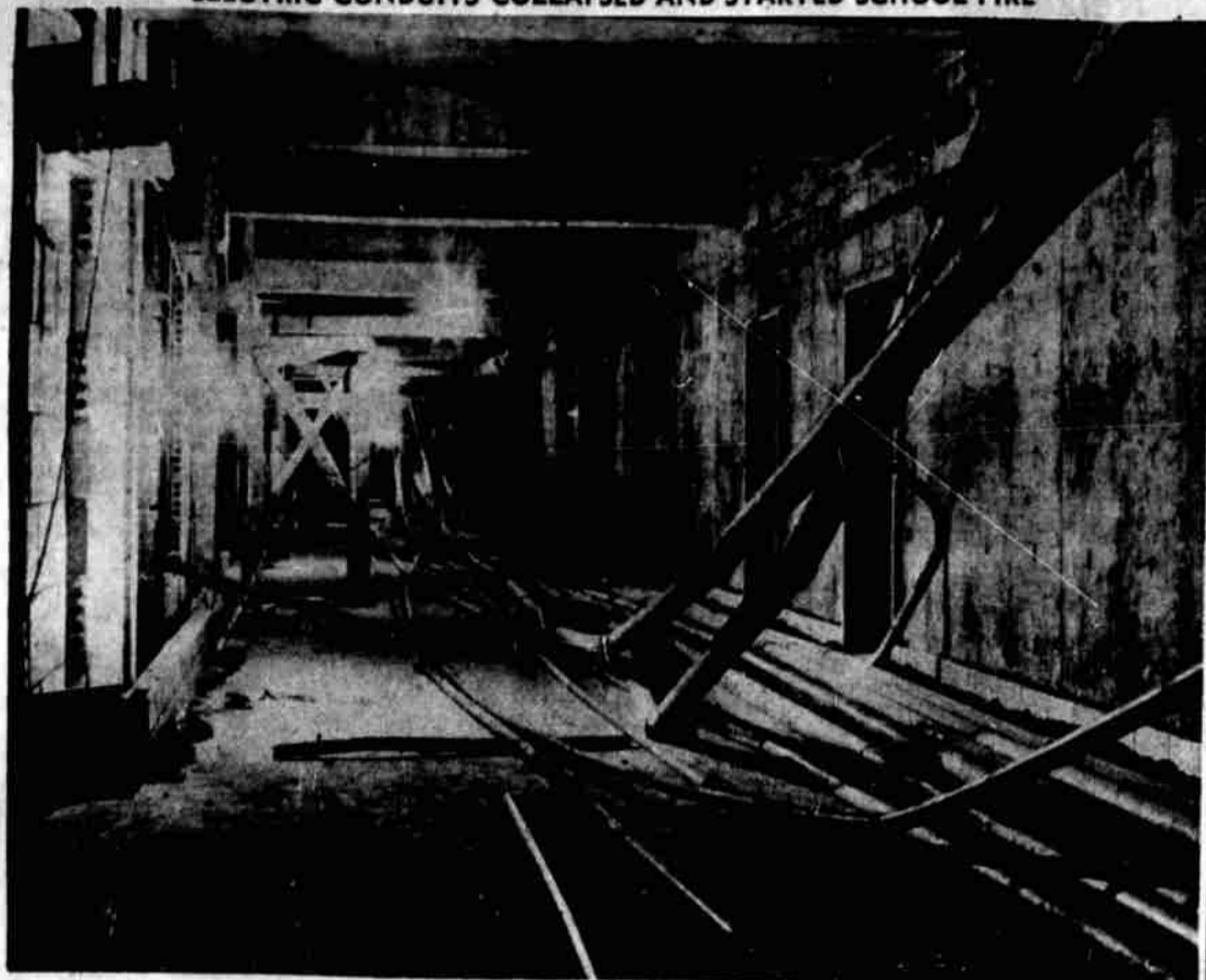
These conduits for electric wiring, temporarily attached to the overhead structure, collapsed and started a short but spectacular fire at the new South Salem high school building. Damage was about $1500.
