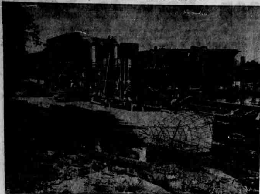
Donald M. Drake, prime contractor for new South Salem high school, employs a large crew efficiently organized to bring Salem's newest and largest high school into rapid completion.
