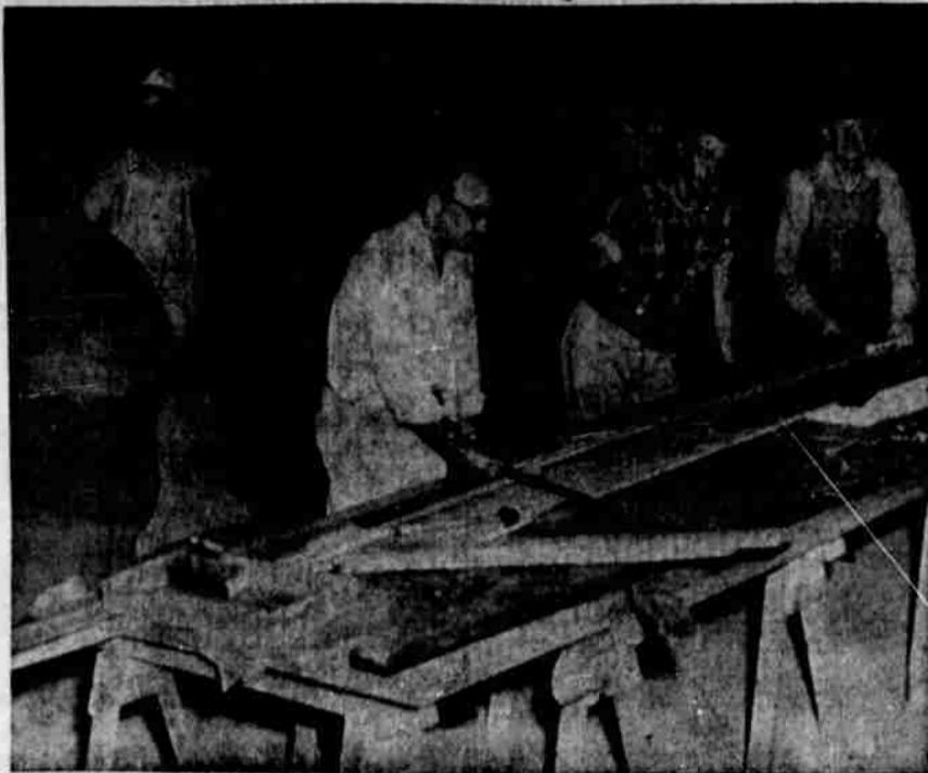
Workmen are putting finishing touches on exhibition booths in the new Polk county fair building at Rickreall. Fair will be held Aug. 28-29-30. From left in photo are County Agent John Hansen, Dean McBee, and L. H. McBee, chairman of the county fair board. In background are Curt Balzer and Tony Kessen.
