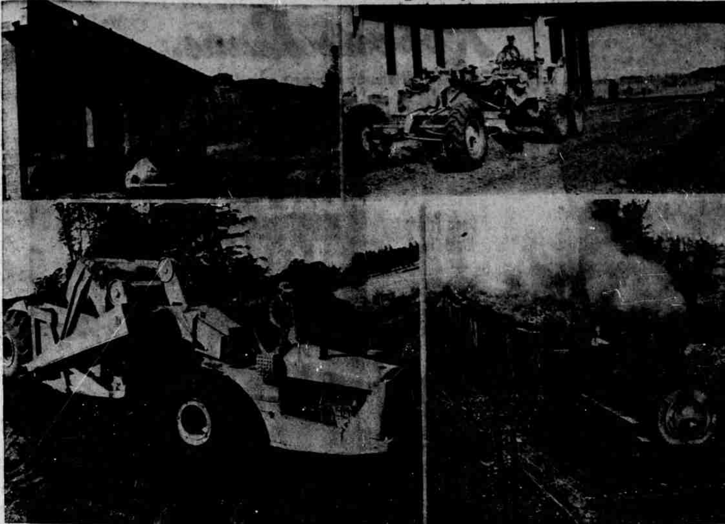
Top, left: Turner road overpass, now standing alone like some classical monument, will join the S. P. overpass when earth now being moved from Bartosz completes the fill between the two viaducts. Lower, left: Ten yard "can" used by Roy Houck, Jr., prime contractor for this section of the by-pass to move about 165,000 yards of earth from Bartosz hill to complete a by-pass fill to Mill creek overflow. Top, right: Grader working in a new nine tenth mile realignment of Turner road that passes beneath the overpass. Lower, right: See the train roll. New overpass spanning S. P. track may become a mecca for railroad photographers because of picture possibilities offered here by track curvature.
