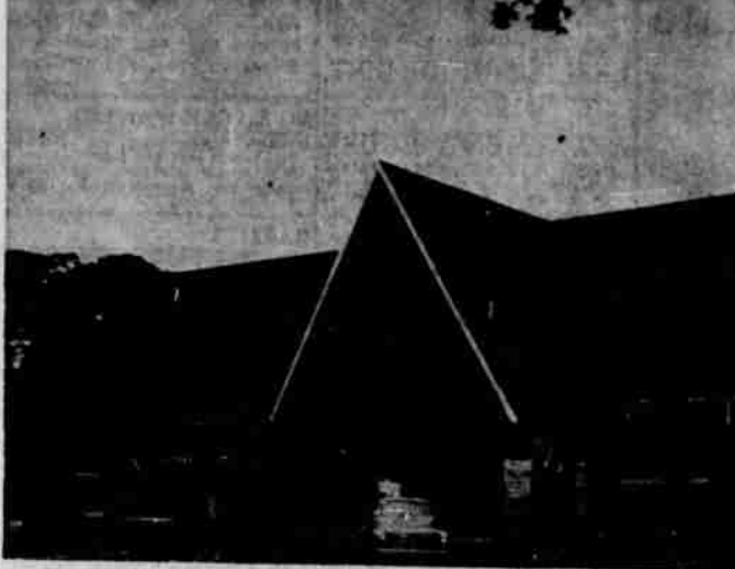
Edifice under construction at High and Myers street for St. Paul's Episcopal church by A. Minden, prime contractor, will be ready for Christmas services if plans of the contractor and James Payne, Salem architect, are realized.
