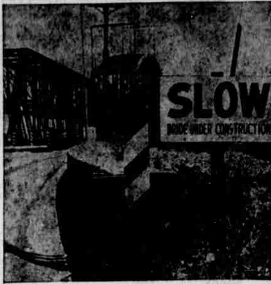
Motorists crossing the Mississippi river on the Lewis and Clark bridge at St. Louis, Mo., can get a good laugh of this sign, if they have a quick eye. The sign, with the letter "G" missing from the word "bridge" refers to a temporary approach being constructed at the opposite end of the bridge. (AP Wirephoto)
