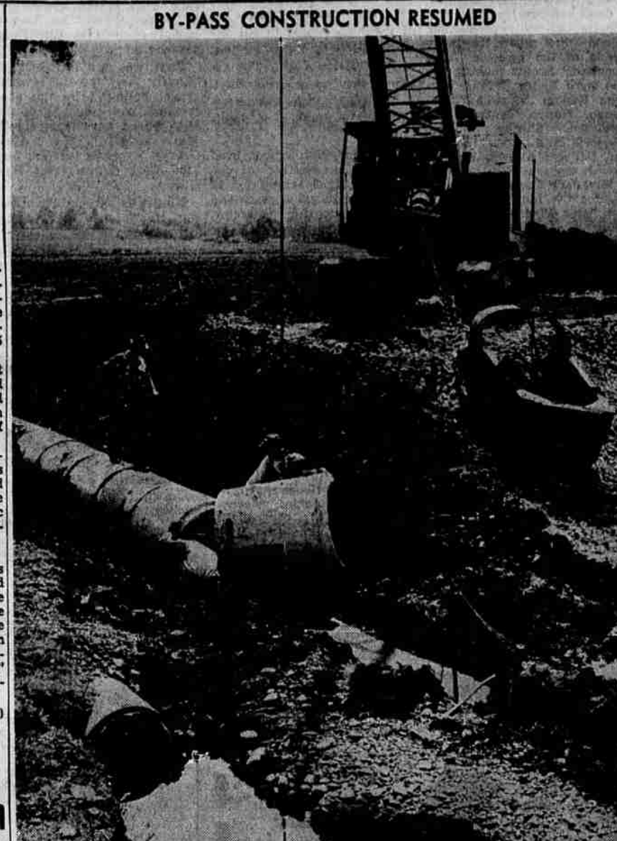
Shown in this photograph is the six man crew of Vernie Jarl, Gresham contractor for a section of the East Salem By-Pass route, placing 36-in culvert pipe across the new route a half mile south of East State street. Jarl and other contractors along the route will begin extensive operations as weather conditions permit.
