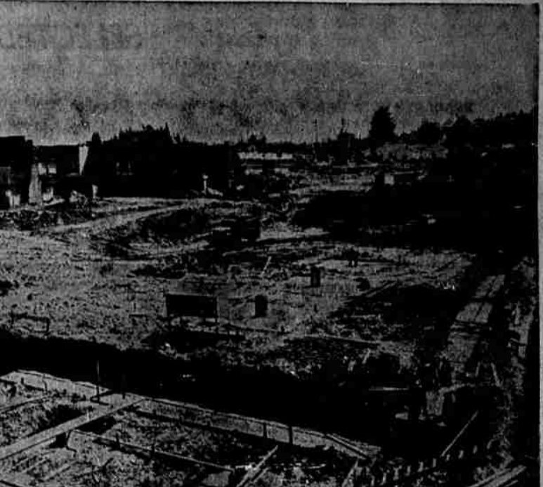
This photograph made from a construction site adjacent to Leslie junior high school shows excavations and construction for new $3,500,000 South Salem high school extended over an area two blocks square.
