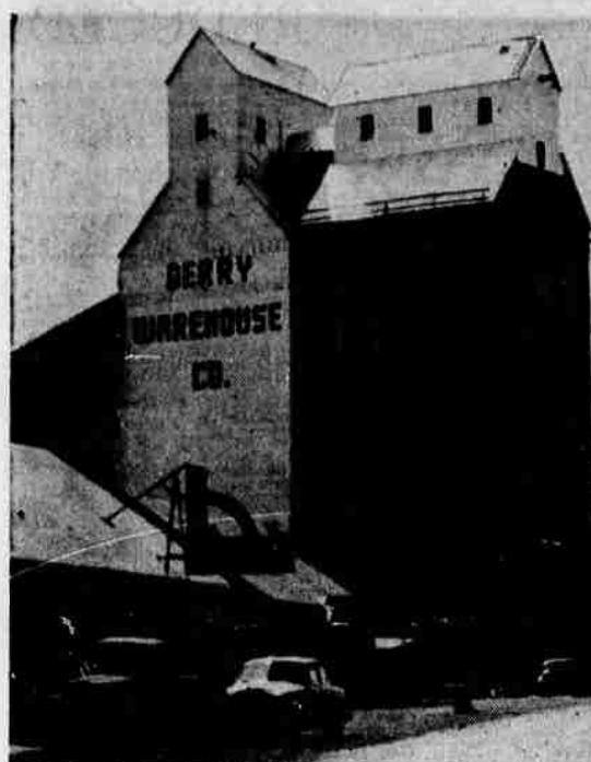
Workers started placing aluminum skin on new 100,000 bushel grain elevator addition being built at Derry by the Derry Warehouse Co., near Rickreall on the Dallas-Salem highway. New elevator will double storage capacity of the plant.
