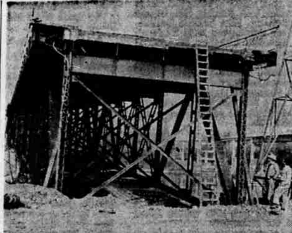
Pondering the Big Lift—Luther Jensen, highway resident engineer and his assistant, Len Wallace, speculate how Moore Drydock company will lift the shore span of the old Center street bridge, estimated to weigh 544,000 pounds, 11 feet three and five-eighths inches. The span beyond, weighing 830,000 pounds, must be raised six and a half feet.
