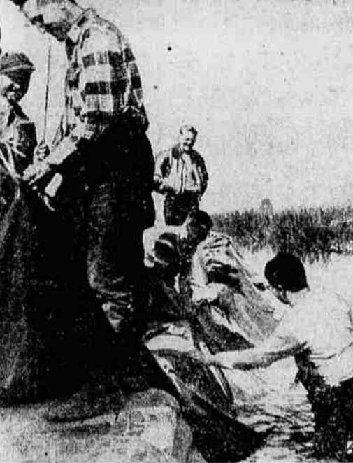
Fighting Floods by the Yard—Amused by a new "wrinkle" in the fighting flood, workers stretch plastic material on the outside of a sandbag dike at Winona, Minn., to prevent seepage. A strip of the material 1,700 feet long and 52 inches wide was stretched along a critical dike that so far has protected Winona from the highest Mississippi river floods on record. (AP Wirephoto)
