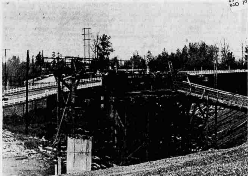
A Look at Things to Come—Shown under construction in the foreground is the grade separation for the new Salem bridge. This separation will extend to the outside lane, now the grade section of the new Riverview highway through West Salem. American Bridge company will make a large concrete placement over longitudinal beams on the grade separation in about 10 days.
