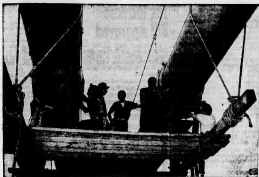
Tightening the Cables —Workmen tighten bolts on the cables of George Washington bridge between New York and New Jersey from a platform that will follow the span.
