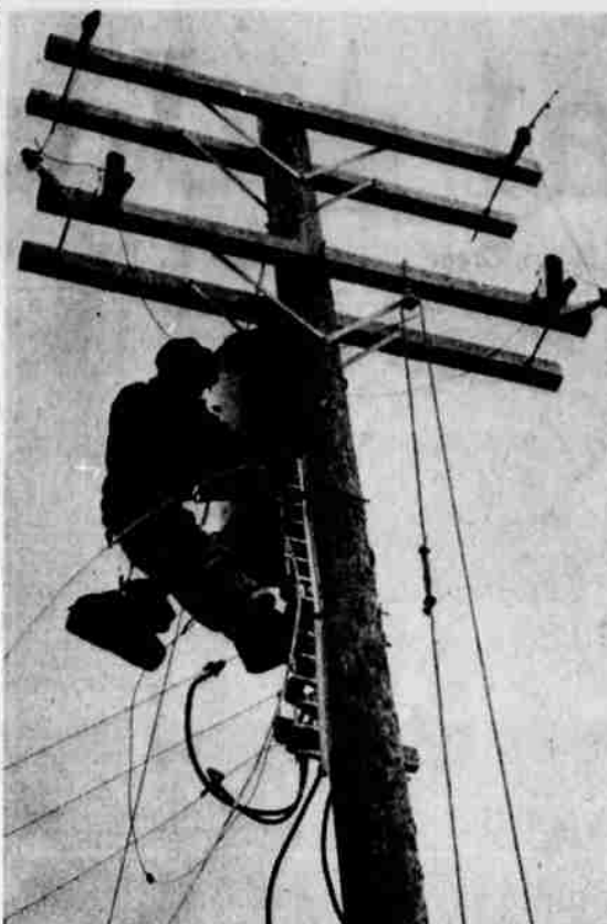
For the Festival—L. E. Bellows, Portland General Electric lineman, is hooking up the lighting for the Cherryland festival at the State Fair grounds. Shown are the 220 and 110-volt wires for the complete lighting of the stage.
