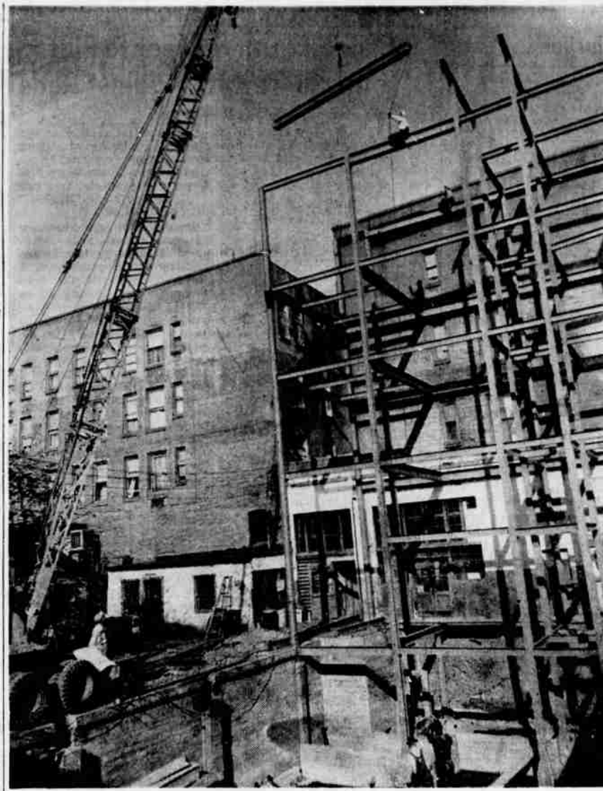
Steel Placed For Senator Hotel Annex—Charles Drake company, Portland utilizing a construction crane with an extension boom places top steel for the five story annex now under way for Senator hotel. R. D. Bruce, steel foreman, states that three seven ton girders will carry the second floor club room and that iron work will require near three weeks for completion.
