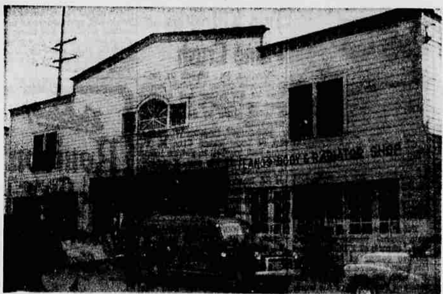
Horse and Buggy Barn Dismantled —Cherry City Feed barn, last feeding barn to operate in Salem, now being dismantled at 540-42-44 Ferry street to make room for a parking lot. Cherry City Feed barn housed about 200 horses and buggies on occasion but was never a livery stable.
