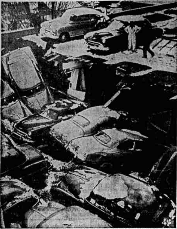
New Cars Come Down —Not the price, but 14 new cars themselves, tumbled down at this Victoria, B. C. agency when the roof collapsed. A salesman escaped by diving beneath one of the eight used cars crushed below. Cause of the collapse has not been determined. (AP Wirephoto)
