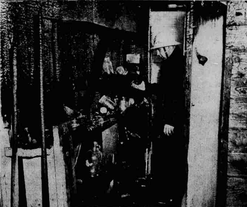
Inspects Fire Damage—Glenn Shedeck, city fireman, inspects damage done to garage of B. O. Bachelor at 1390 Hoyt street in a Saturday morning fire. Bachelor was not home at the time of the blaze but a next-door neighbor removed this auto.
