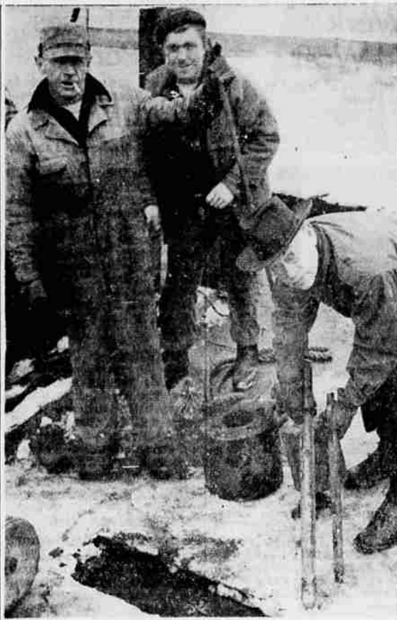
Ready to Probe Foundation Formations—A. C. Thomas (left) foreman for Raymond Concrete Pile company and E. G. Ricketts (right), state highway bridge investigating engineer, who holds halves of a Gow sampler spoon to be used in investigating earth structures at the site of Willamette bridge piers.
