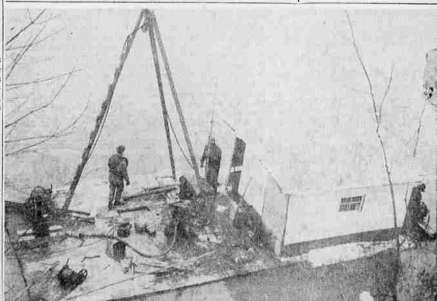
Work Starts on New Willamette Bridge Site—Barge containing equipment for exploring earth formation at the bridge pier locations moves into position at the foot of Marion street to sample subsurface structure at the site of pier number two.
