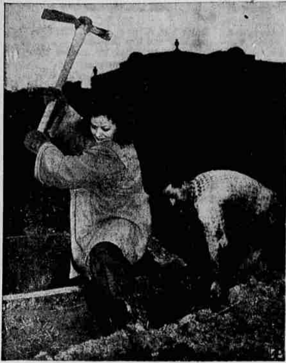
Does a Man's Job—Mrs. Margaret Pallas, 22-year-old divorcee, swings a pick in digging a trench on a building construction job at Chicago. She takes turns in an eight-hour day digging trenches, mixing cement and carrying tile pipe, receiving a $10 daily wage. She had tried office work for a year, but gave up when she became ill. Behind her is her boss, Donald Buss, 31, a contractor, who says he and Mrs. Pallas intend to get married. She has a two-year-old daughter who is cared for by relatives during the day. (AP Wirephoto)
