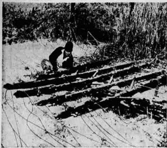
Winter Wonderland?—Working in a wonderland of ice and a maze of wires, telegraph groundman Arthur F. Kenney, Jr., seemingly has a bewildering job ahead as he repairs telegraph pole snapped by weight of ice which formed during sleet storm. Kenney was one of the many linemen called out to restore disrupted power and communication facilities in wake of storm which struck Sedalia and other Missouri towns. (Acme Telephoto)
