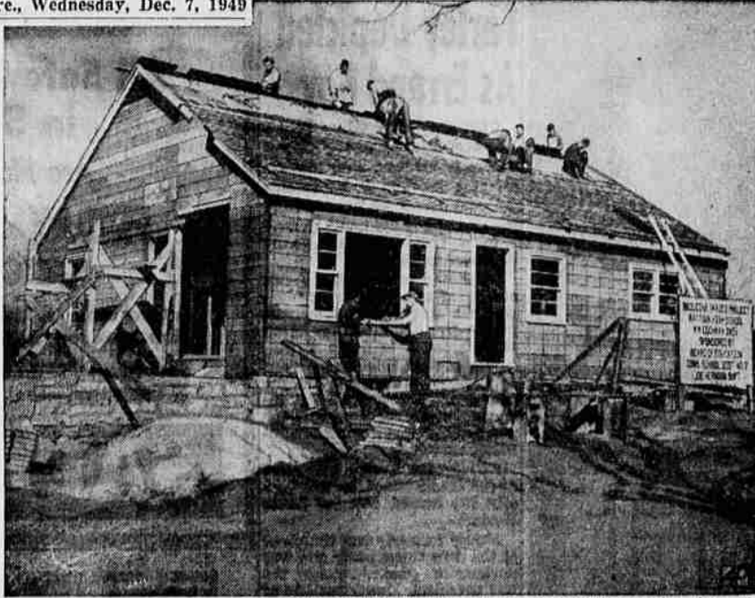
Student Project—Students in the building trades class of Raytown, Mo., high school, work on the six-room house with garage they are building as part of their class work.
