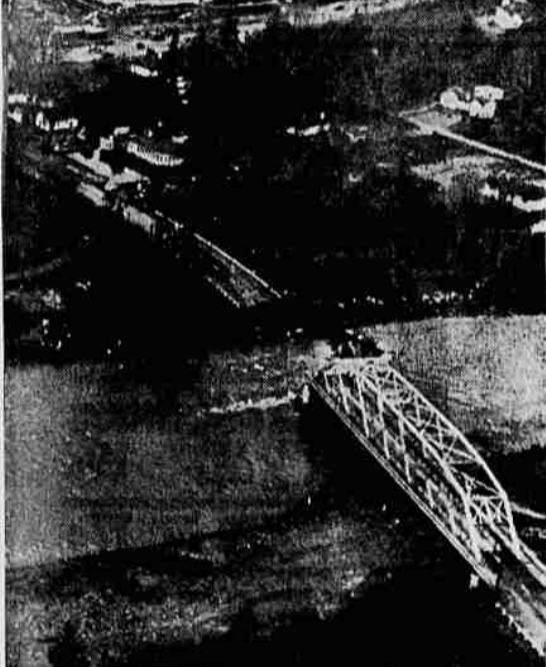
Storm Washes Out Bridge—One of the heaviest storms ever to hit the northwest washed out a 200-foot span of the Capilano river bridge at Vancouver, B. C., and virtually isolated the community of West Vancouver. The storm left 28 persons dead, hundreds of homes flooded and untold millions of property damage as it roared over the Pacific northwest states. (Acme Telephoto)
