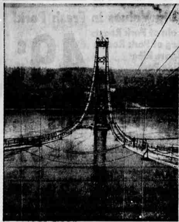
Sky-High Bridge Work —Five hundred feet above waters of Puget Sound at Tacoma, Wash., workmen move around narrow catwalks during construction of $13,000,000 suspension bridge. In background is one of span's two 508-foot towers. Bridge will replace the first one called "Galloping Gertie" a few miles northwest of Tacoma which collapsed almost nine years ago.
