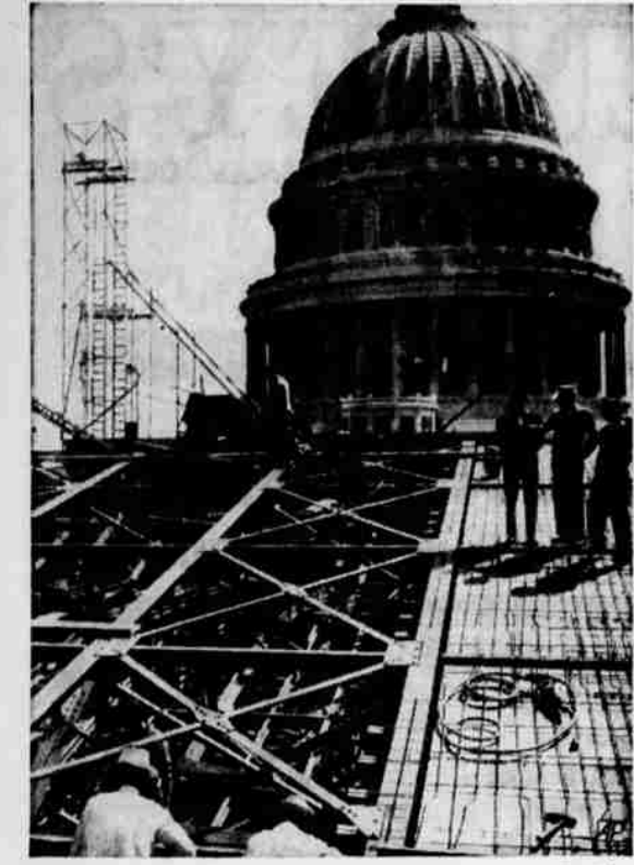
Roof for Senate—Joseph Duke, sergeant-at-arms; David Lynn, capitol architect; and Sen. Dennis Chavez of New Mexico (left to right) inspect new senate roof in Washington.
