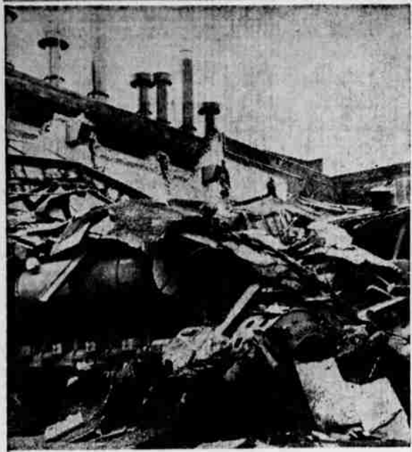
Blast Wrecks Power Plant —Turbine room of a million dollar power generating plant in Rushville, Ind., lies in ruins after a diesel engine developed a hot piston and blew up. Two men were killed in the blast. The plant provided electricity for 11 counties. (Acme Telephoto)
