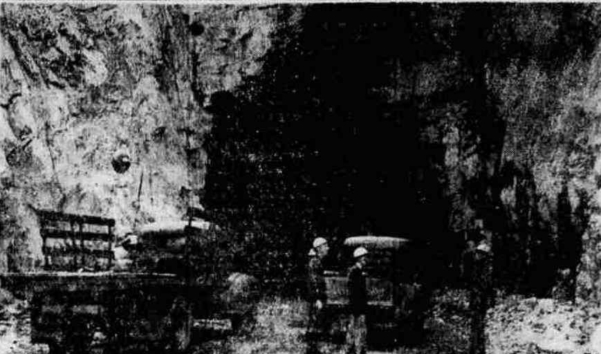
Scenes at Detroit Project—Top, viewing westward from this vista point east of Detroit dam is a panorama of the construction area. Old and new highways are shown at the right as well as a great cable anchor now under construction above the highway. Access roads on the left bank of the North Santiam lead to the stone quarry. Center: Here, at Detroit damsite, is the marshalling yard of Consolidated Builders where heavy construction machinery is being assembled for use in expediting dam building. About 500 men are now employed at or near the damsite. Below: West portal of the diversion tunnel through solid rock which is progressing at a rate of about 45 feet daily. About 550 feet of rock remains to be excavated and waters are being taken that the job will be completed before September 10.
