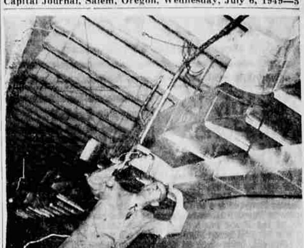
Cool Air for Hot Legislators —William E. Healy, assistant secretary of state, examines ducts now being installed to air condition legislative committee rooms on the second, third and fourth floors of the capitol. Air will be cooled by four compressors with a capacity of 100 tons of ice daily. Installation costs will amount to about $50,000.
