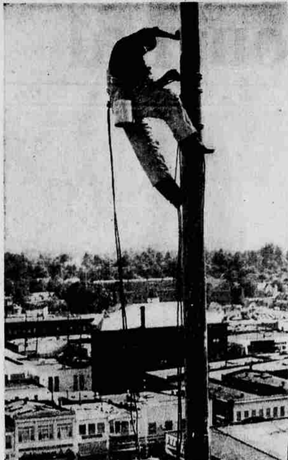
As the Flagpole Painter Views Salem—W. R. Cox, veteran Portland steeplejack, coats in the flagpole on the Livesley building more than 100 feet above the street. Two coats of paint will be applied with caulking between coats.
