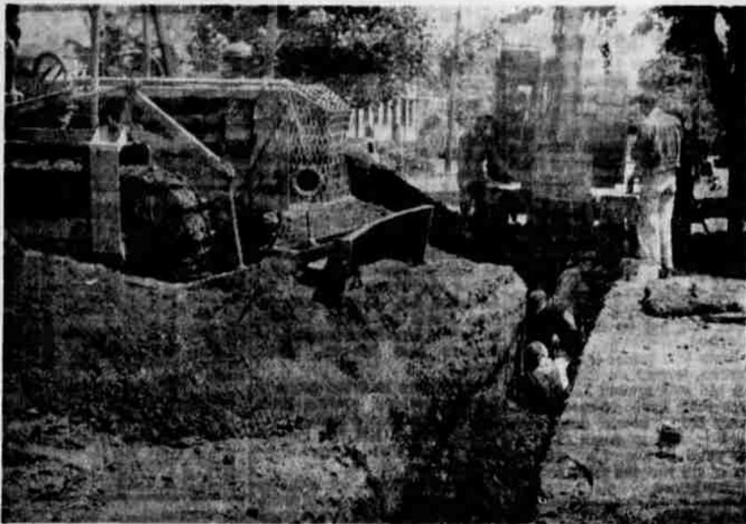
Dallas—A crew of the Salem Sand & Gravel company is at the end of the line with the new 16-inch main from the site of the city's new three million gallon reservoir. The job of laying the line is now completed but for cleanup work. In the above photo men are shown cutting into the Main street line at the Clay street intersection. (Abel Photo).
