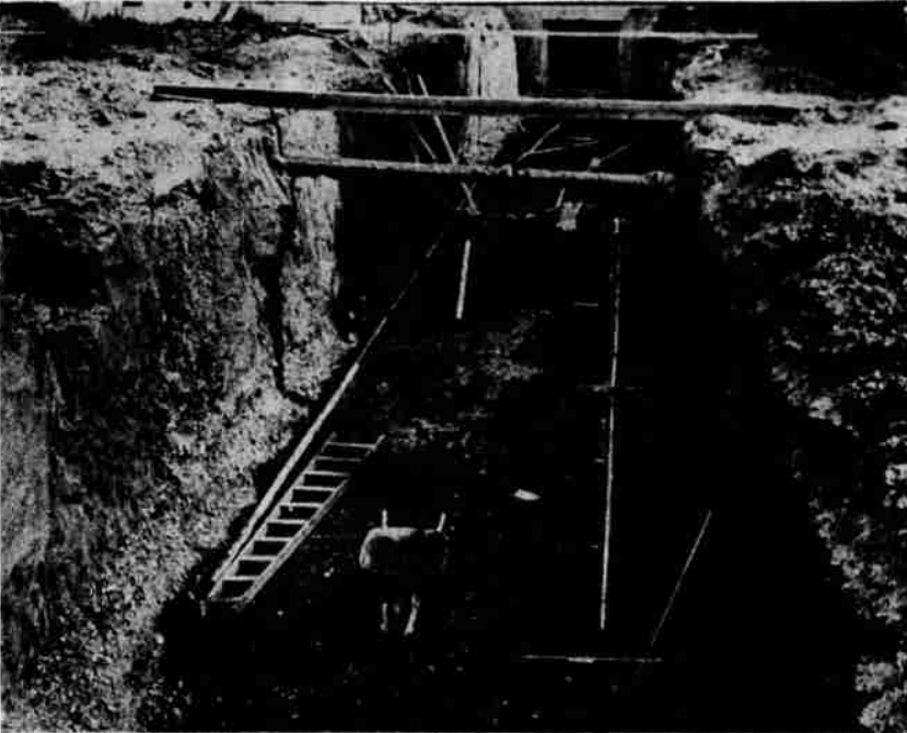
Excavation Accomplished for Access Tunnel —Access tunnel between new state office building and capitol is now complete in respect to excavation across Court street 11 feet deep and 18 feet wide. Next week forms will be started for concrete to form ceiling, floor and sidewalls.
