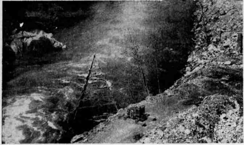
Hydro-Electric Development Starts at Big Cliff —Engineers make soundings at site of Big Cliff power dam where generators operating from Detroit dam spillways will ultimately develop 100,000 kilowatts. Completion date for this project and Detroit dam is set for 1953.
