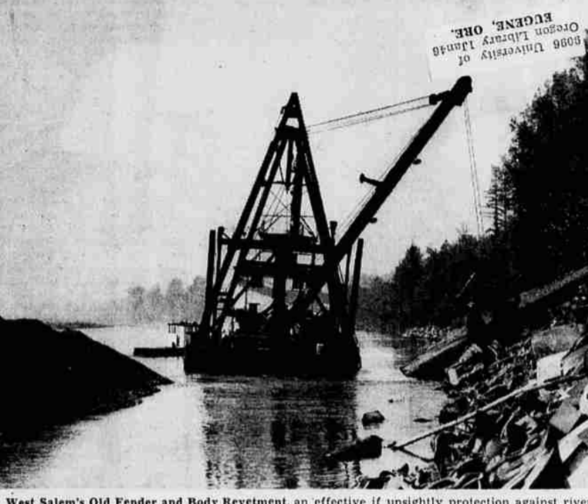
West Salem's Old Fender and Body Revetment, an effective if unsightly protection against river erosion, is now being covered with gravel spread by the U. S. engineer's dredge, Monticello.
