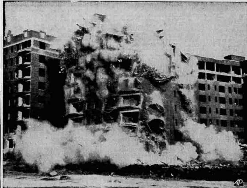
Apartment House Blasted to Provide for New Building—Washington, D. C., was subjected to a planned "bombing" when one wing of the $2,000,000 Boulevard apartments was dynamited to make way for the $4,000,000 first unit of the proposed $26,000,000 war department building. This picture was made just as the dynamite exploded and the walls of the nine-story building began falling. — Associated Press Photo.
