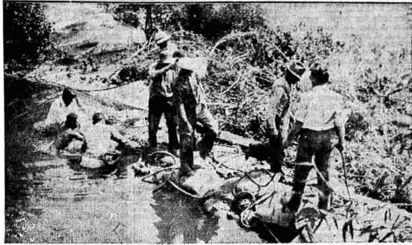
More than 300 men were mending a break in the San Joaquin river levee near Modesto, Calif., with sandbags to prevent further damage to truck gardens. Hundreds of acres have been flooded with an estimated damage of $150,000. (Associated Press Photo)
