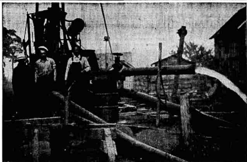
Silverton—Silverton was assured of a water supply for years to come this week when its new well was tested and found flowing 750 gallons a minute. This is the city's first well. Heretofore Abiqua and Silver creeks have furnished the supply.
