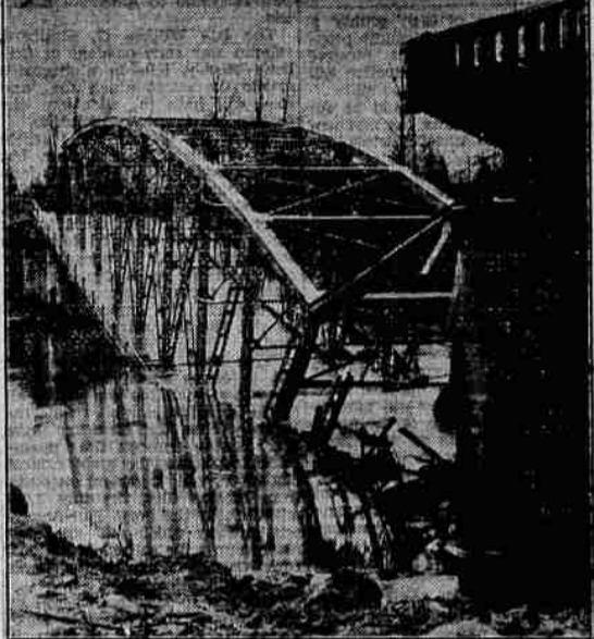
A blazing gasoline truck stalled on the Snoqualmie river bridge east of Seattle, Wash., generated so much heat that the steel span shown above was melted. The driver jumped into the river, escaping with slight burns. (Associated Press Photo)
