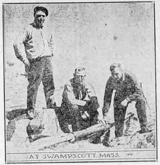
So that President Coolidge may stay aboard the yacht Mayflower and still keep apprised of the happenings of the day, men are laying a cable from the "Summer White House" at Swampscott, Mass., to the anchorage of the vessel in the harbor.
