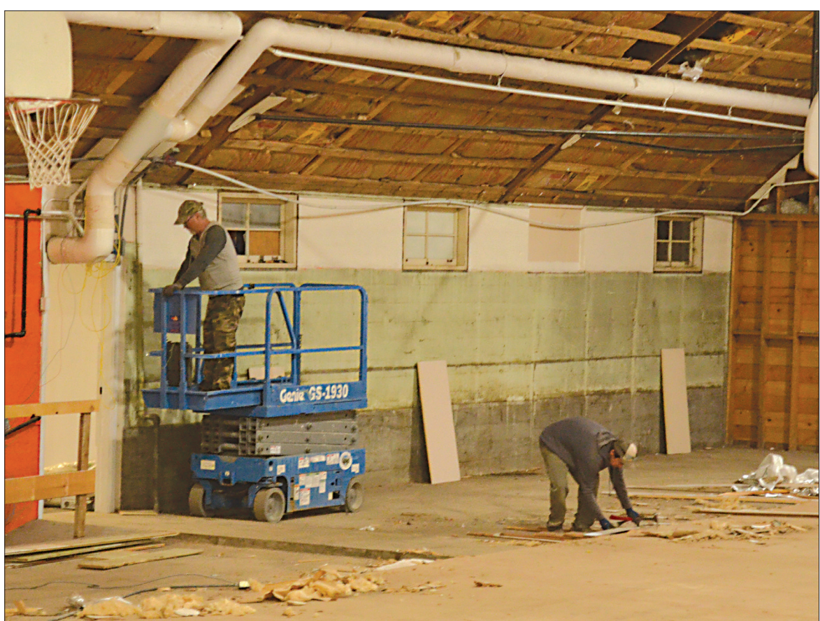
Workers clean up Thursday, March 17, 2022, during the demolition work at Wallowa High School's Cougar Dome. It's part of the work toward the seismic retrofit the school district received a grant to pay for.
