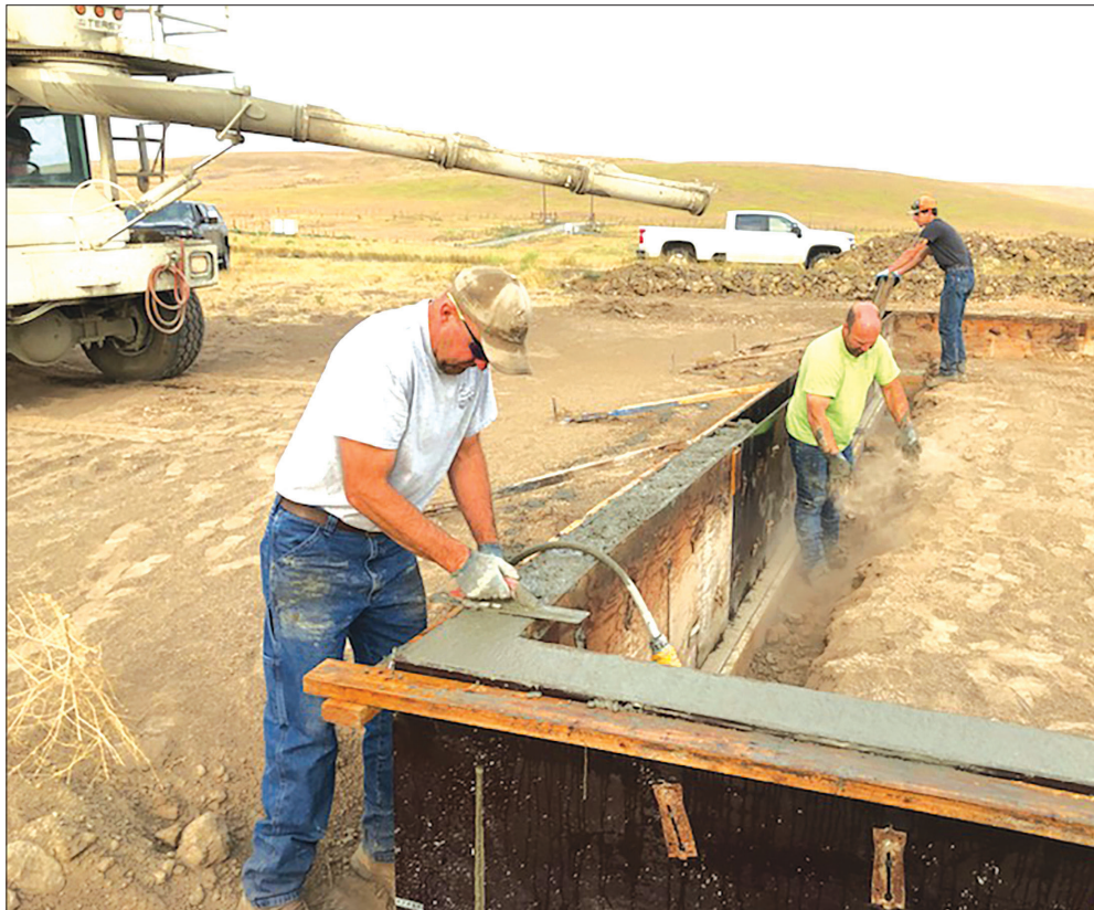
Work has been ongoing on a new multipurpose educational building at the Eagle Cap Shooting Range north of Enterprise. On Thursday, Aug. 5, 2021, workers poured the stem walls. From left, are Donnie Rynearson, Curt Huston and Aaron Eggart, while John Harris operates the truck and spout.
