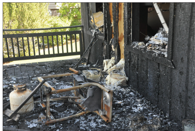
A damaged grill lays on the deck of the Griffiths' Enterprise home, with a Little Chief Smoker, which the Griffiths said was the source of the fire, laying behind it.
