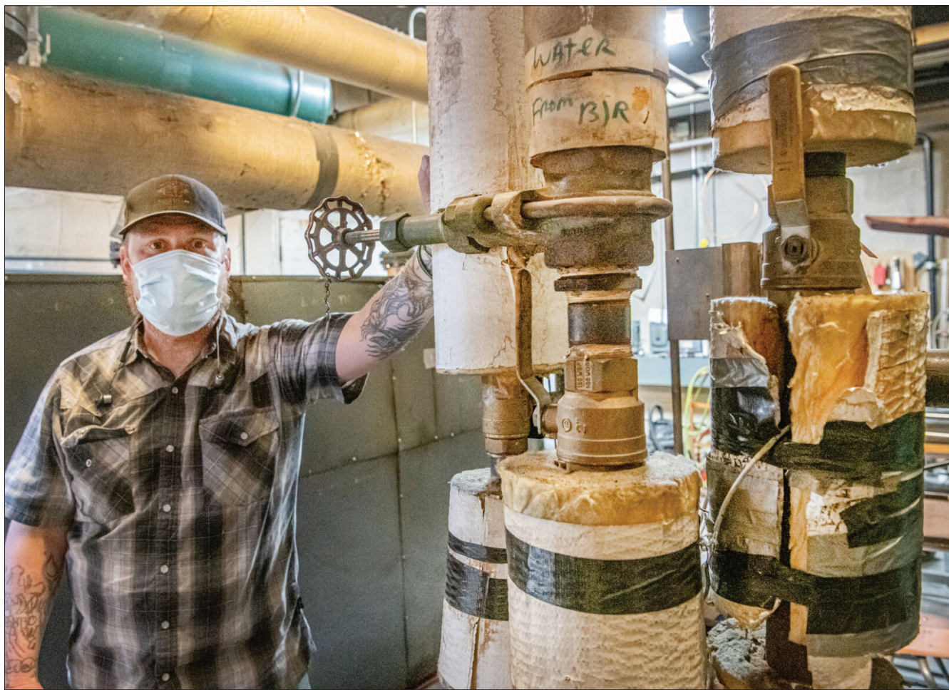
Wallowa School District maintenance head Jake MacDonald stands next to pipes that carry hot water through the school buildings for heating. The heating and cooling systems are among those in the district in need of improvement, and that improvement is on the way thanks to Wallowa voters passing a $7 million bond during the Tuesday, May 18, 2021, district election. The bond passage also means the district will get a $4 million grant from the Oregon Department of Education.
