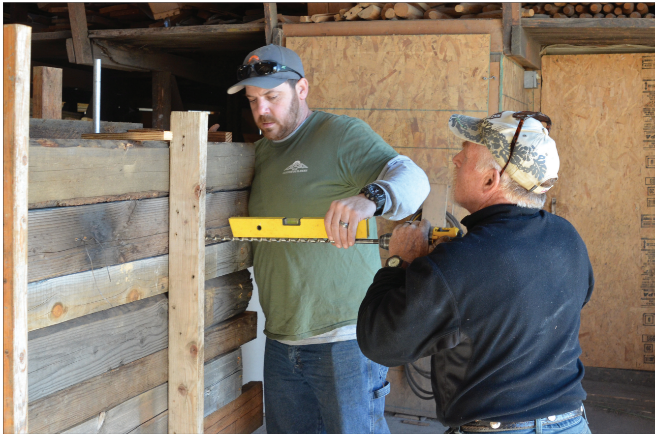
Marty Weber, left, co-owner of BLH Custom Builders, helps carpenter Kurt Klages on Friday, March 26, 2021, on a mock-up for a house the company is building at Wallowa Lake. The former Bronson Log Homes has expanded to constructing conventional-style homes as well.
