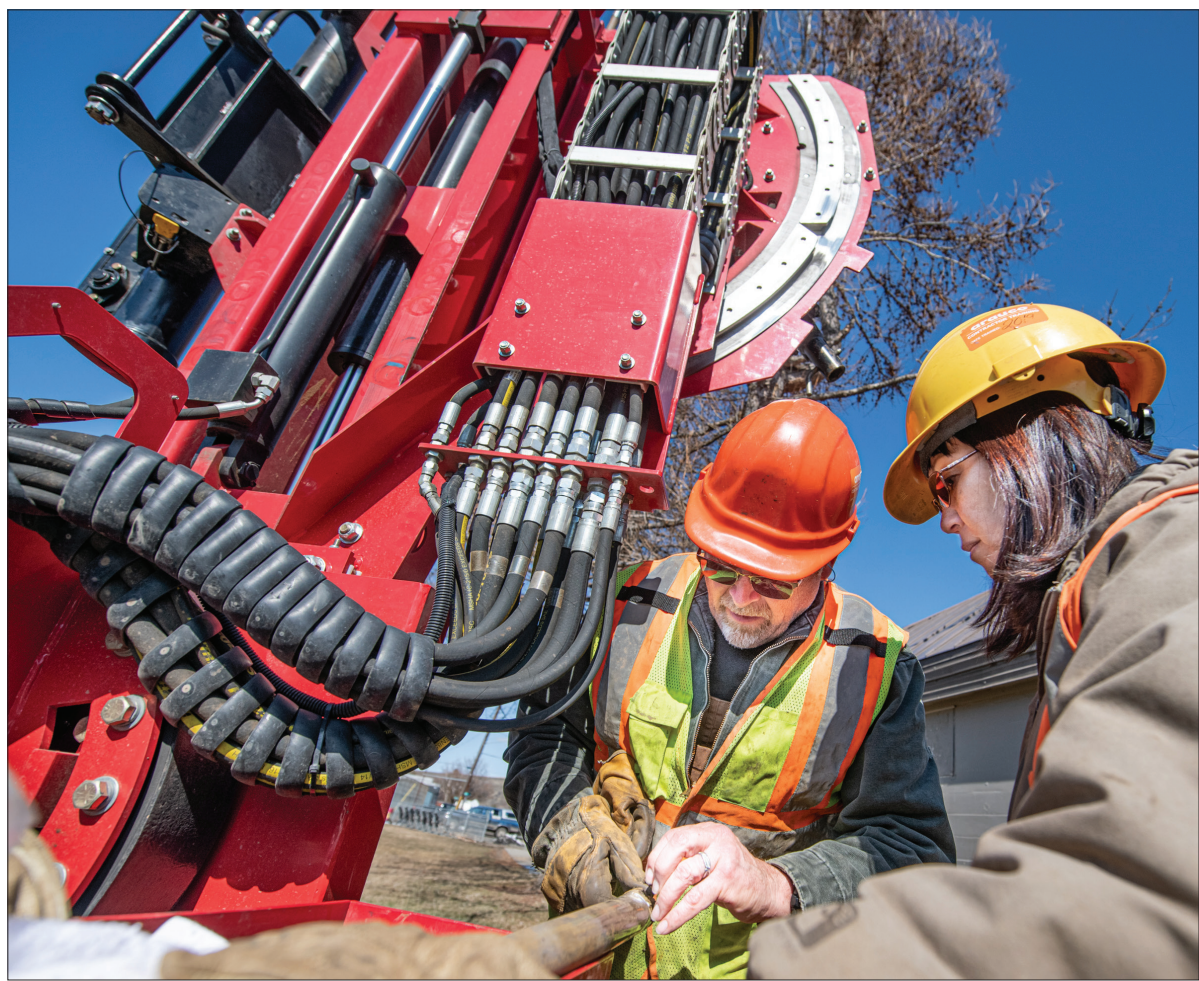
Ellen Morris Bishop/For the Wallowa County Chieftain Geotechnical drillers Michael and Marvis Remboldt examine a core sample they drilled on the west side of the Wallowa High School Cougar Dome on Tuesday, March 16, 2021.
