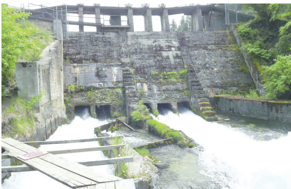
Until Wallowa Lake Dam is repaired, its impoundment can only be filled to 72 percent of storage capacity.
